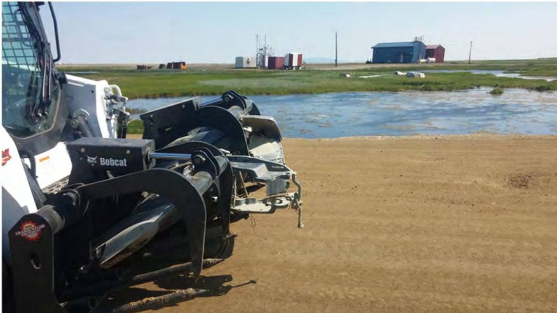
(With the multiple attachments solid waste issues that goes beyond the landfill was getting the treatment too) *illustrated here is the grapple forks picking up an old motor to be disposed
