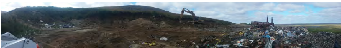
(A clear workface is one of many BMP's for a landfill and with resources pulling together to get a handle on it was the city of Scammon Bay pulling cover material from within the landfill the bobcat was able to move the dirt throughout the landfill
