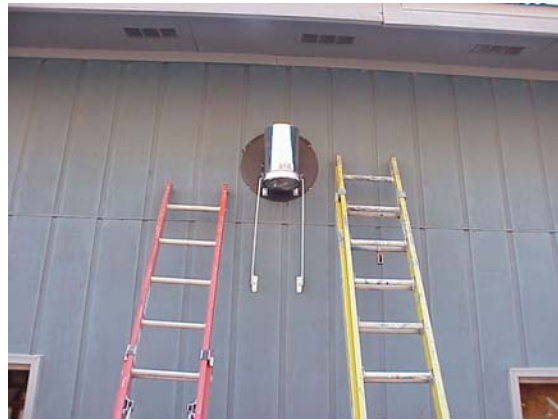
Stack coming out of the building
