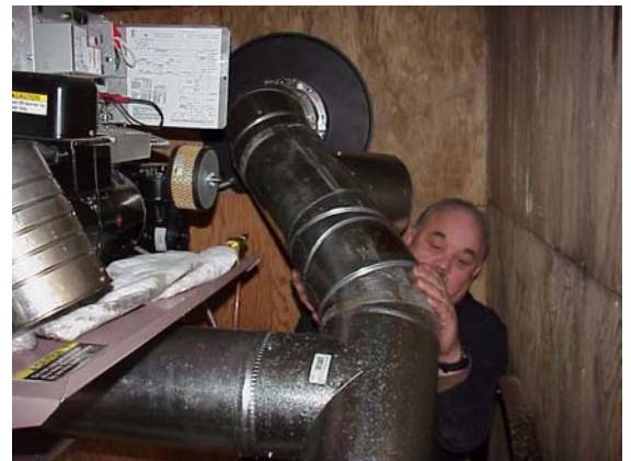
Another example of a stack being fed to the outside of the building from another used oil burner
