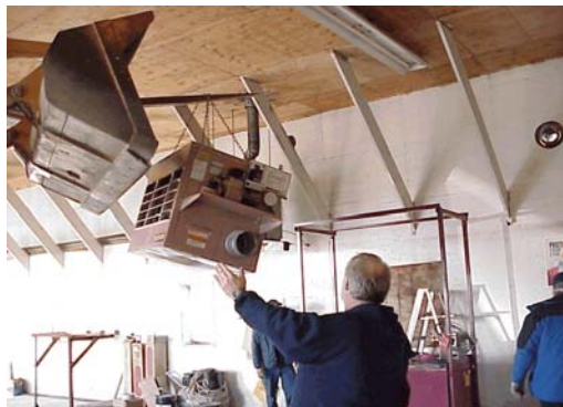
Heavy equipment being used to lift heater unit onto the used oil burner
