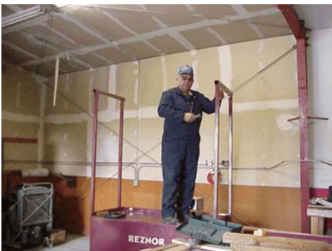
Starting the installation of a used oil burner at Goodnews Bay (Dennis Lundine, DEC)
