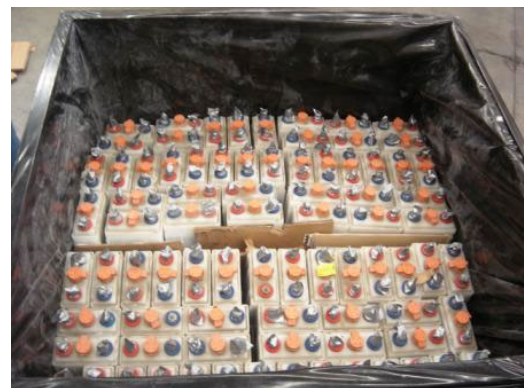
Batteries with cardboard inserted between them for better stability
