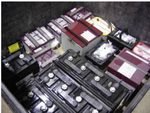
A completed first layer of lead acid batteries
